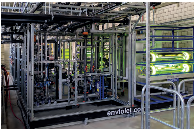
Figure 19: UV-skid of a continuous wastewater treatment plant placed at an API manufacturing site.
