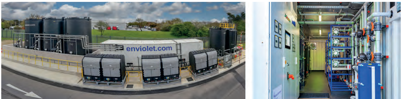
Figure 18: Continuous wastewater treatment plants at CMOs for CIP-rinse wastewater from API formulation with a max. of 200 m 3 /d, overview (left) and inside view (right) of the treatment container.
