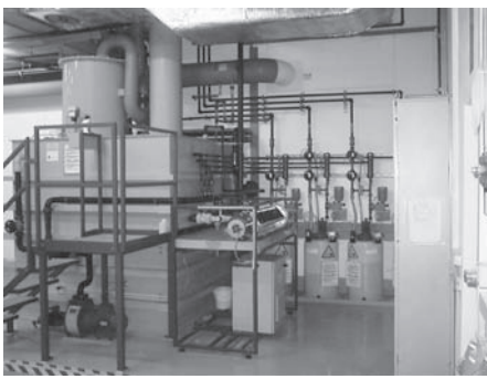
Figure 2. The treatment plant for the detoxification of Cu EDTA at Multek, completely delivered and installed by a.c.k.
