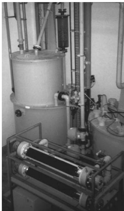
Fig. 5: CyanoMat®; front left 24kW Enviolet UV-reactor, back left treatment container for the principal oxidation with gas cleaning, back right treatment tank for pre-oxidation with integrated process technology
