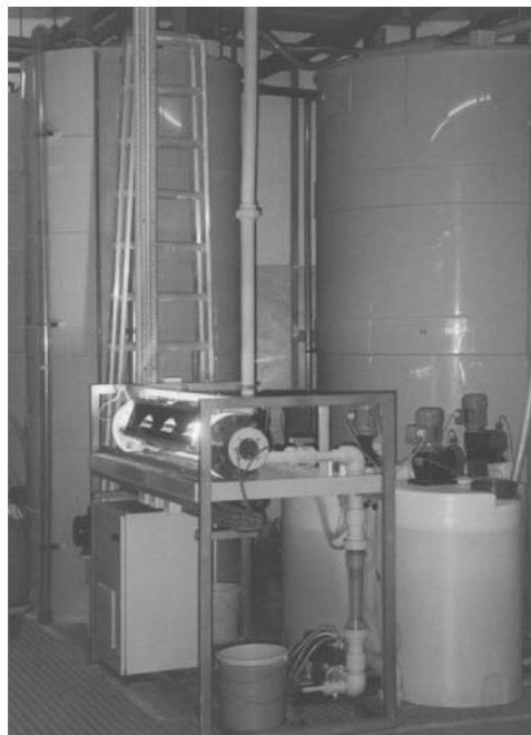
Fig. 3: Enviolet ® UV-reactor in CyanoMat ® -system at Binder
